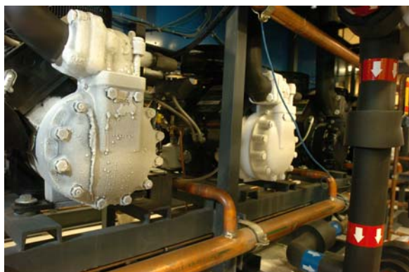
Figure 2 : Suction by low-temperature compressors
